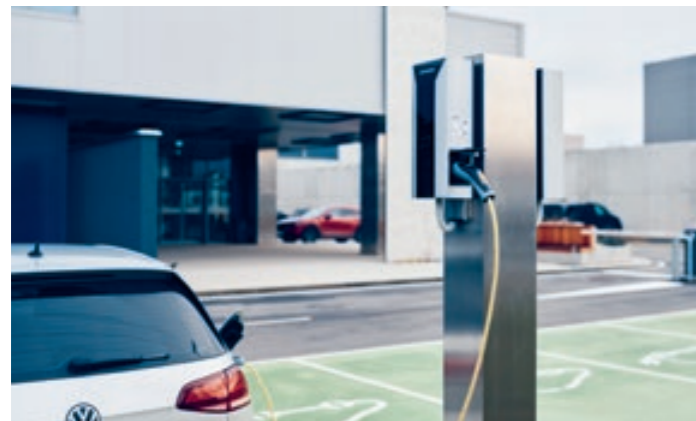
Sustainable development: The charging stations for the company's vehicle fleet are powered by rooftop solar panels.
